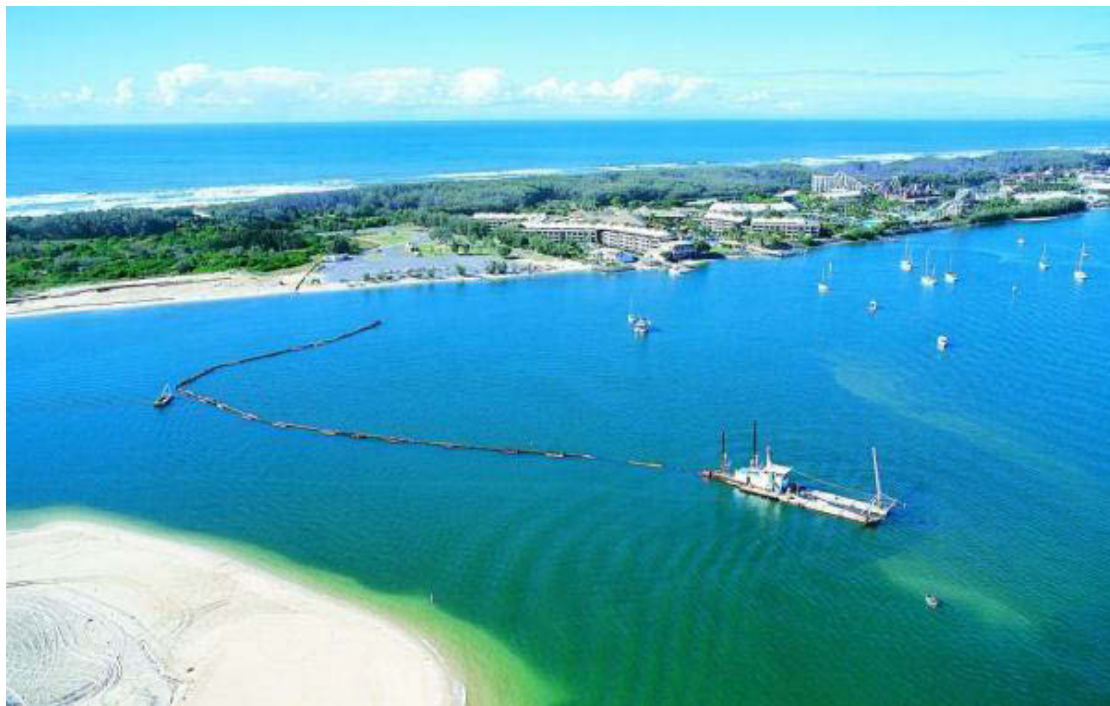
Figure 4 Sand dredging as part of the Northern Beach Protection Strategy. Source: Neumann Contractors www.neumanncontractors.com.au
